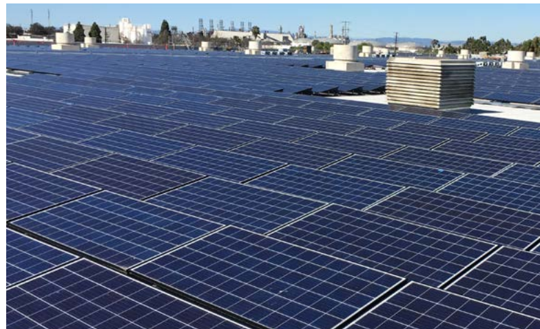
Honda installed one of Southern California's largest corporate owned on-site solar arrays.
